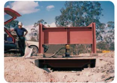
Force being tested and calibrated at site with the portable test unit
